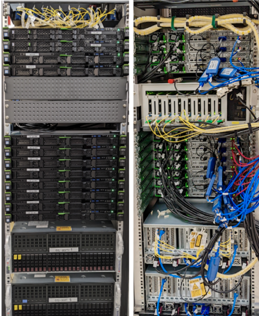
Figure 5.7: Photos of the ACA Spectrometer installed in the ACA correlator room (Credit: ALMA ESO/NAOJ/NRAO). Major components of the ACA Spectrometer were installed at four computer racks that have been used for the ACA Correlator. The photos show the front (left) and back (right) sides of the computer rack labelled “quadrant 0”, respectively. Two ASMs (one is a working server and the other is a spare server ASMs) and two ASCs (one is a working server and the other is a spare server) are installed at the bottom and upper sides of the rack, respectively. An optical splitter is installed at the most upper side of the rack. Each of the other three computer rack contains an ASM, an ASC, and an optical splitter.
