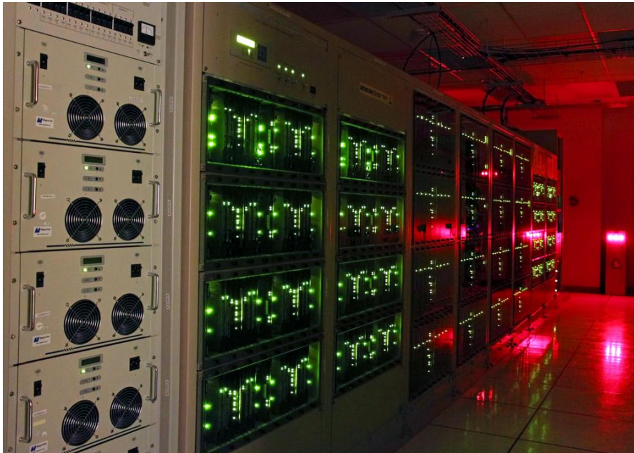
Figure 5.1: The ALMA 64-input Correlator. This view shows lights glowing on some of the racks of the correlator in the ALMA Array Operations Site Technical Building and shows one of four quadrants of the correlator. Credit: ALMA (ESO/NAOJ/NRAO), S. Argandoña
