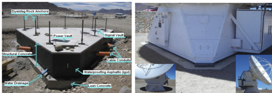
Figure A.2: Structure of an antenna pad (actual pad at the OSF) (left) and detail of antenna anchored to a pad (right).
